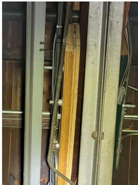
Top Chord Heel at North West side, no split rings
