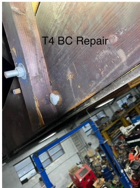
Improper bolt install, and no split rings
