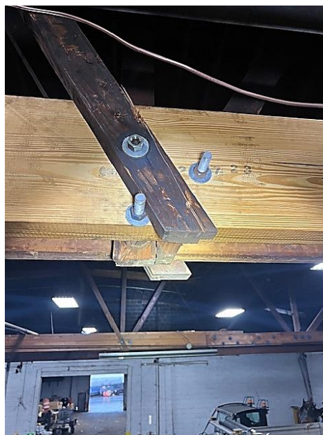
Improper bolt install, split web member and no split rings
