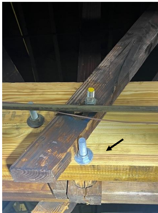
Bolt connection too low in BC member
